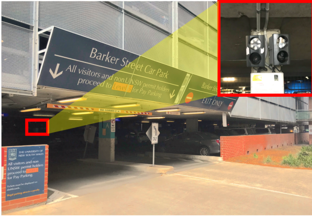
Fig. 2. A real picture showing entrance and exit of our campus car park and a pair of LPR cameras installed side-by-side close to the ceiling of the car park ground floor.
